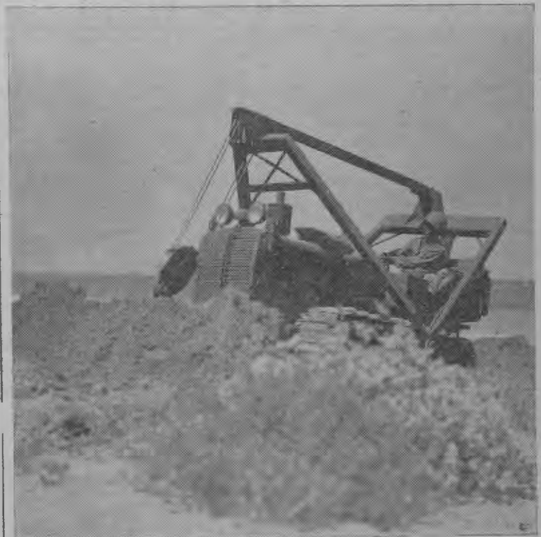
This bulldozer immediately began gouging gun emplacement after coming ashore from LCT during recent amphibious operations demonstrations here. The bulldozer is used in numerous ways after beachheads are established.
